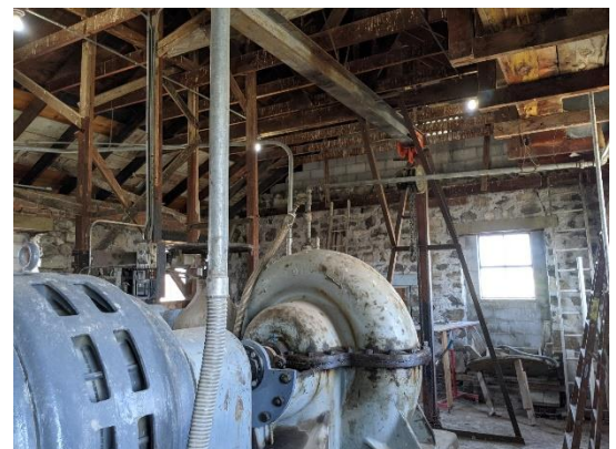
Clover Main Pump House
